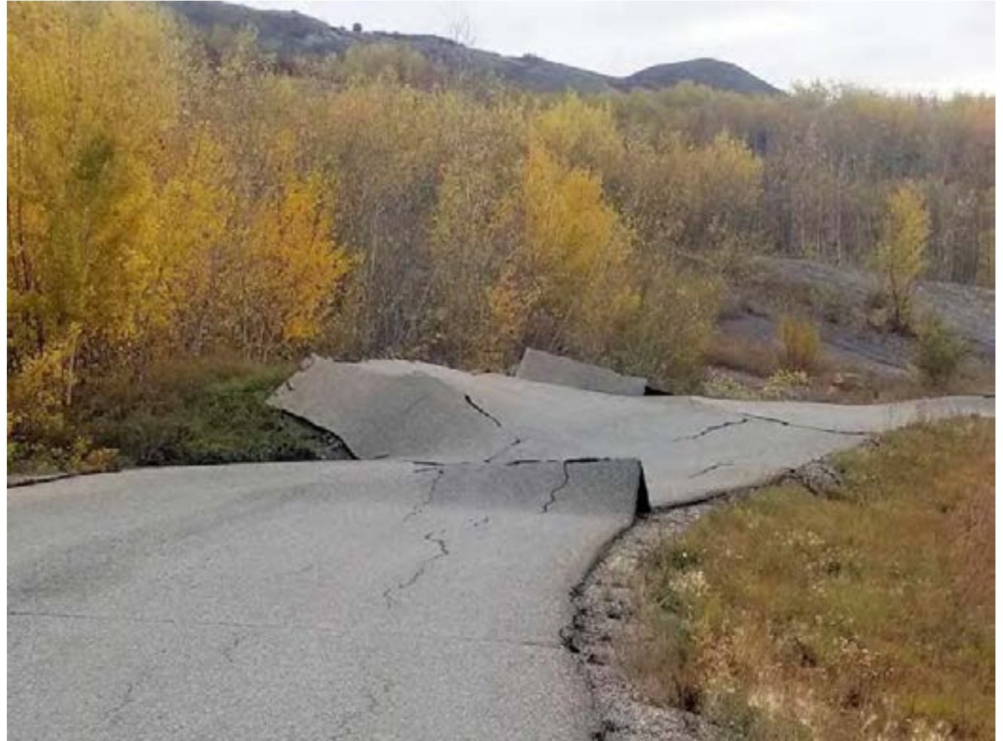
Slow moving landslide impacted road. Credit: YRB North Peace Ltd.
